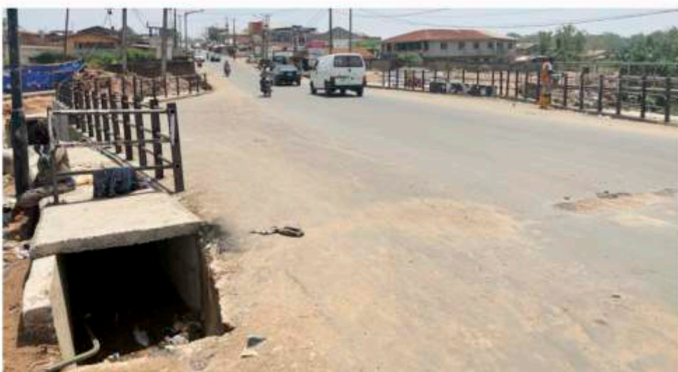
ID 132 (1-Cell Culvert on Abepe Stream near SAMOG along Apete-Awotan Road) after completion
